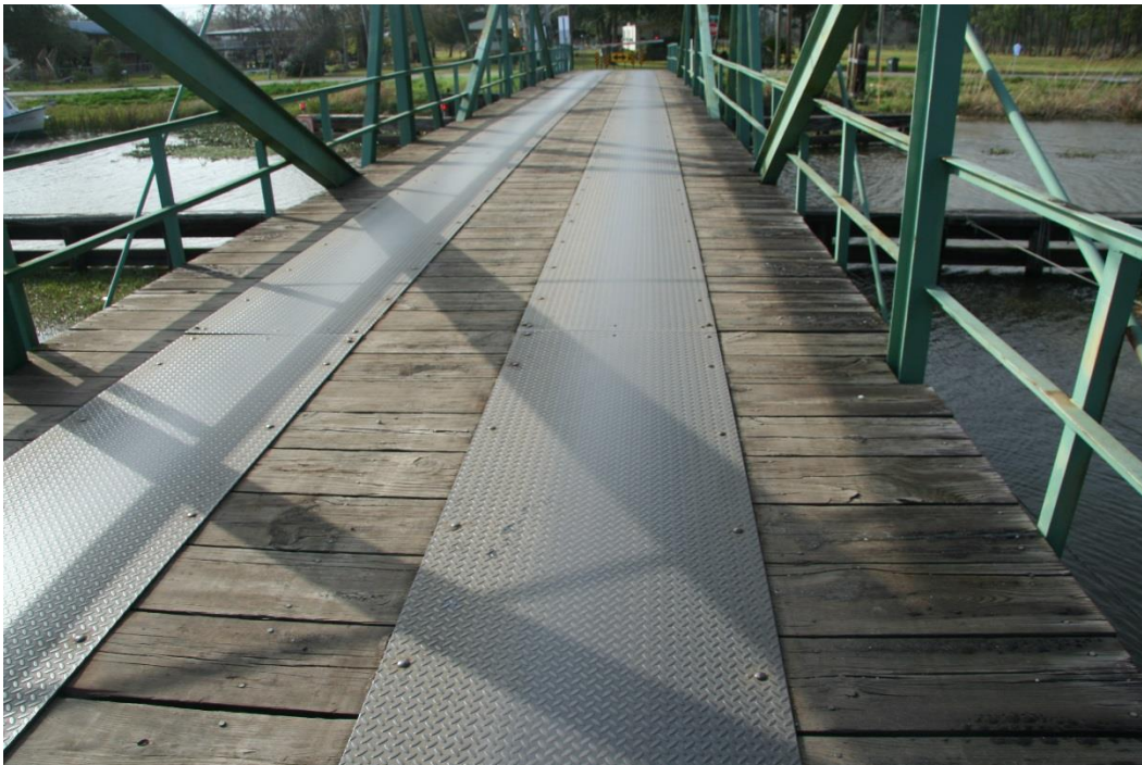
Condition Photo 4: Deck (steel running plates and timber planks) on swing span.
