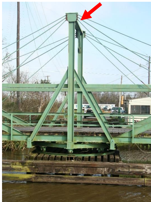
Character-defining Feature Photo 3: Design and construction of a tower structure with cables above the central pivot pier. The cables, along with the top horizontal members added in 2001, support the weight of the bridge when it is in the open position.
