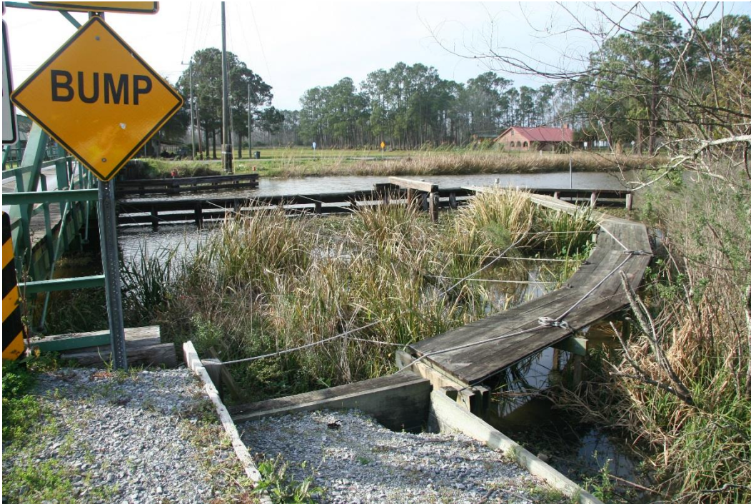
Condition Photo 13: Condition of timber stairway and gravel path to access timber plank platform for the ropes and pulleys of the bridge operating system.
