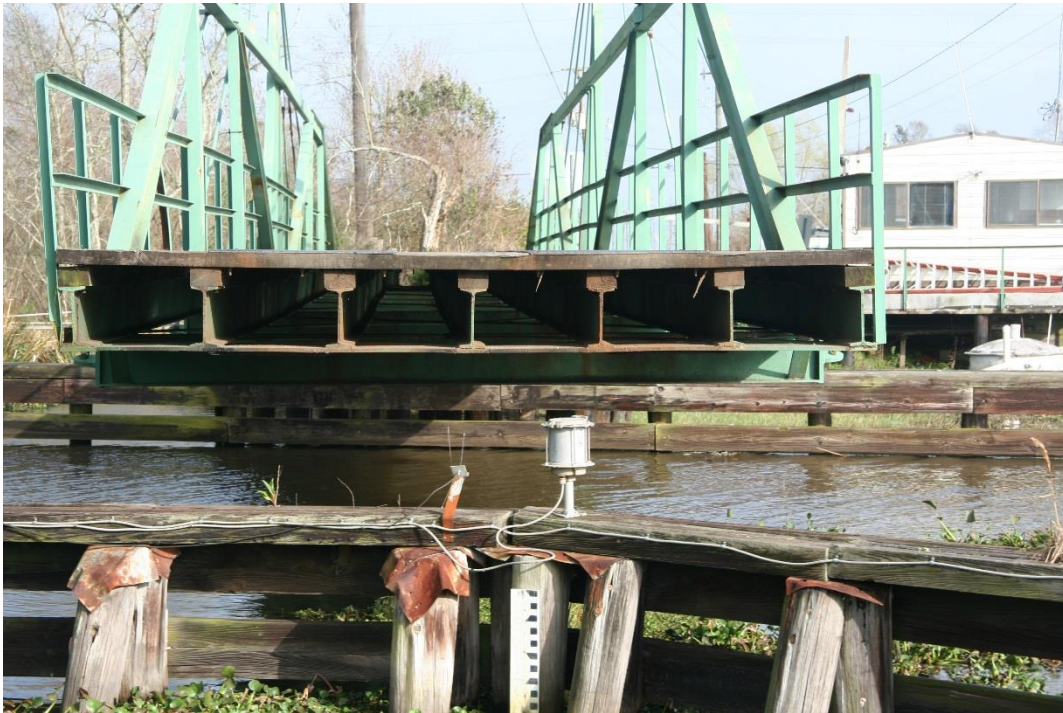
Historic Fabric Photo 1: Steel I-beam floor system on the main swing span.
