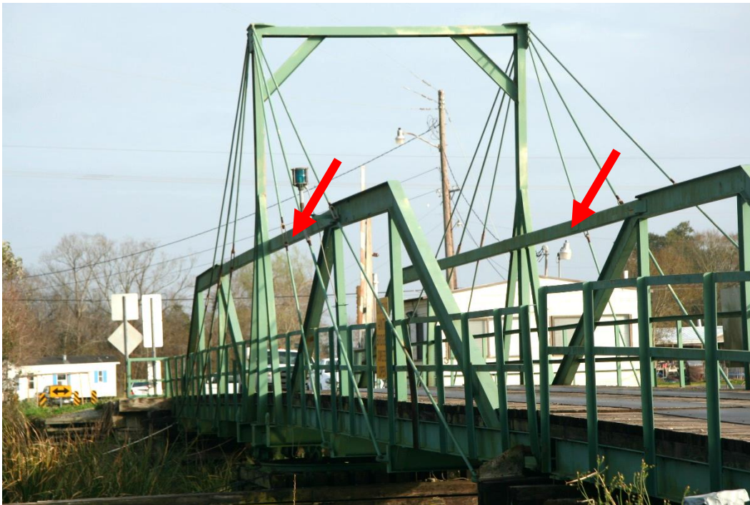
Condition Photo 10: Profile of swing span. Horizontal top chord members on each truss are new from 2001 rehabilitation.
