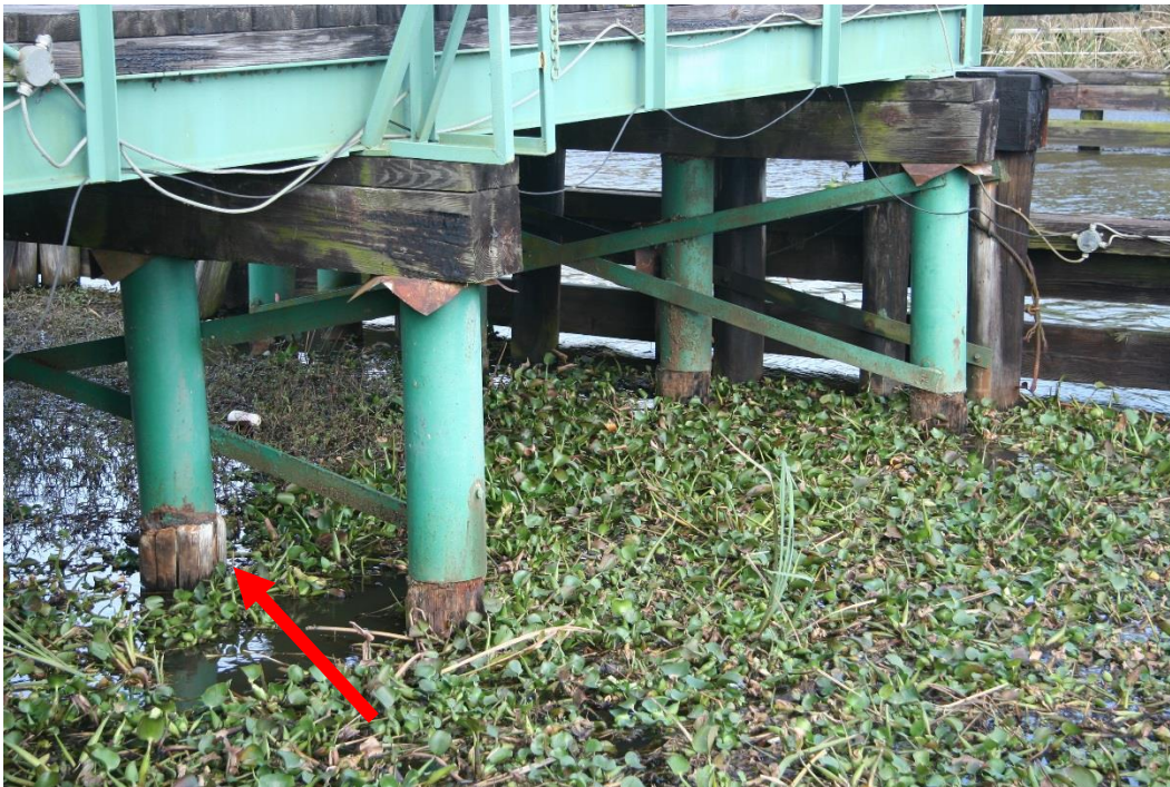
Condition Photo 8: West approach span superstructure and substructure. Note deteriorated condition of timber piles and metal circular jackets for pile splices.
