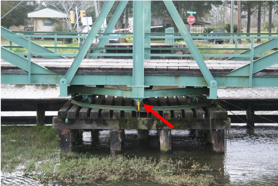
Character-defining Feature Photo 2: Design and construction of center-bearing turning mechanism. This roller-and-track system guides the motion of the bridge when it opens and closes.
