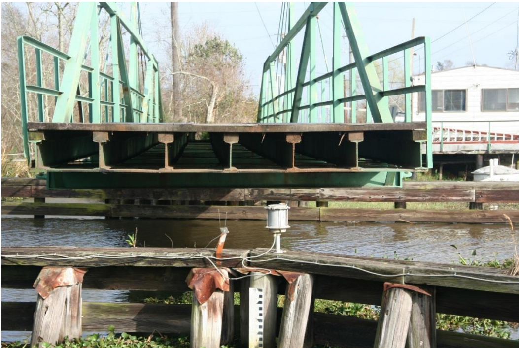
Condition Photo 6: Swing span deck cross section, shown while the bridge is opening.
